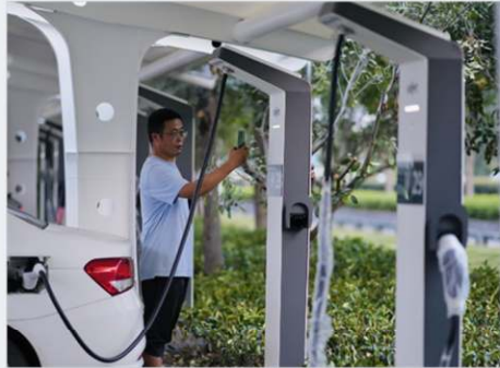
Quzhou Citizen Football Stadium GPC Charging Station
