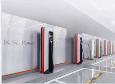
Ningbo Nanyuan Universal Hotel HPC V3 Charging Station
