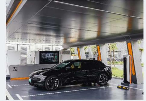
VRMET Electric Wind- PV-ESS - Charging Demonstration Station
